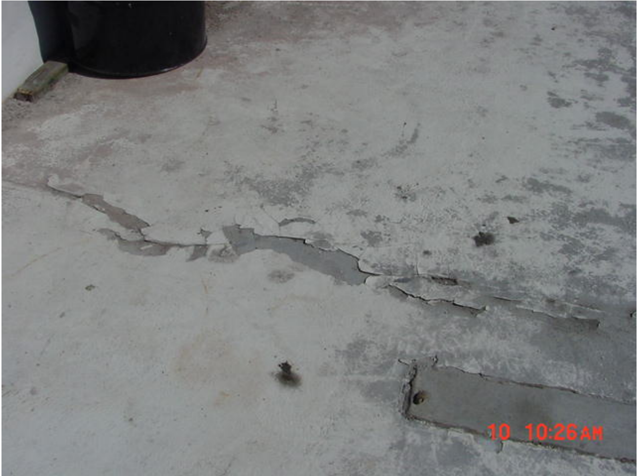
Floor sealant cracking and peeling off of floor and is not providing required protection.
