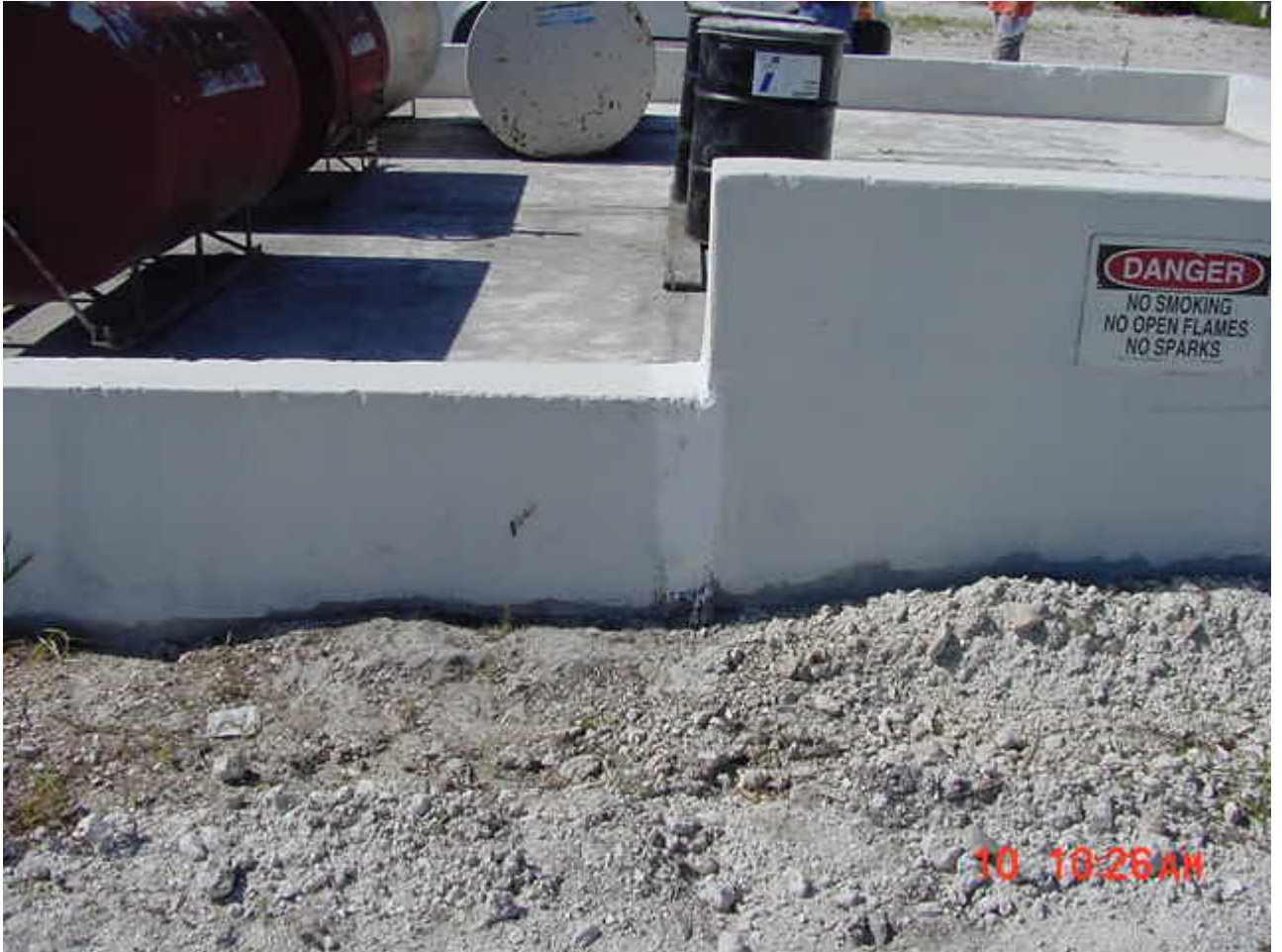
The paint line for the “sealer” does not extend past the floor/wall line. Not sure what type of material was used, but appears to be textured latex paint.
