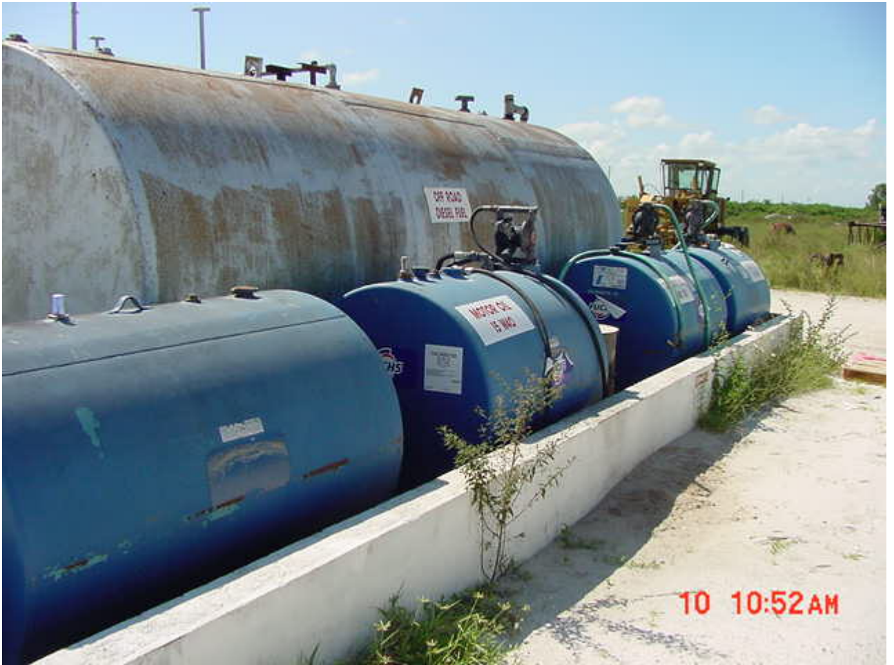
Fueling area along west wall of containment system reveals petroleum discharge.
