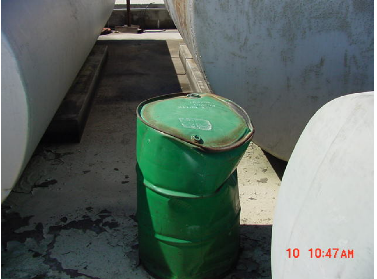
Most of containment system has evidence of petroleum discharges. A damaged barrel of unknown contents sits within containment system on the unsealed floor. System is not protected from the weather.
