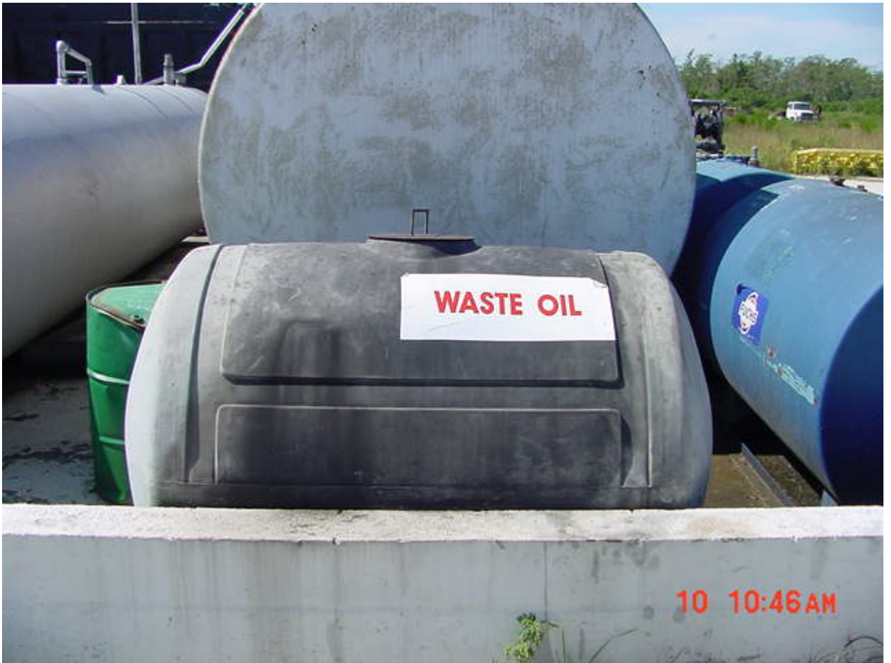
An improperly labeled tank of used oil within an unprotected from the weather, not properly sealed containment system.
