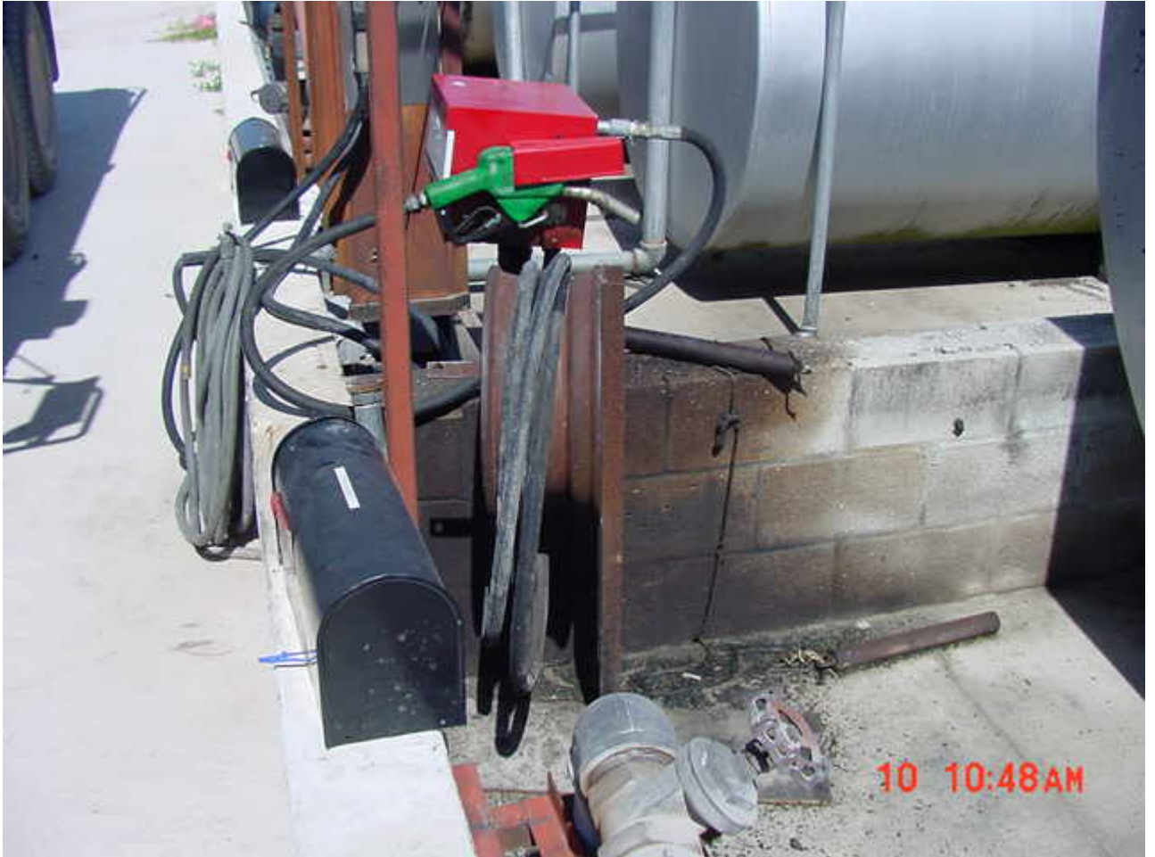
Fueling operation's which reveal sloppy use that contributes to rainwater contamination within containment system. Containment system is not properly sealed and has a drain with unknown ending.
