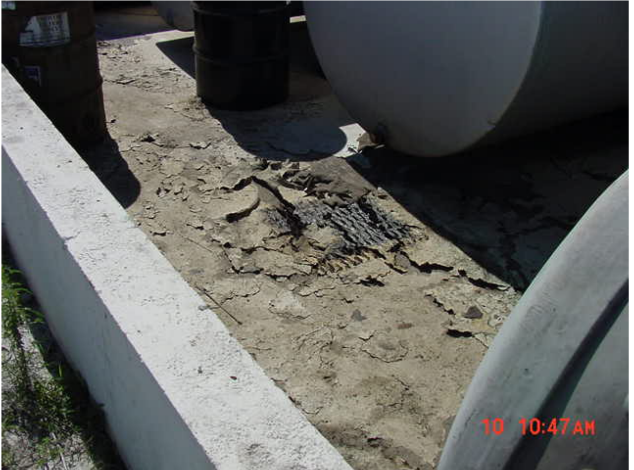
Drain within the containment system shows evidence of petroleum discharge. An algae mat possibly formed from diesel covers most of the containment system floor. Unknown where drain's end or where it goes.
