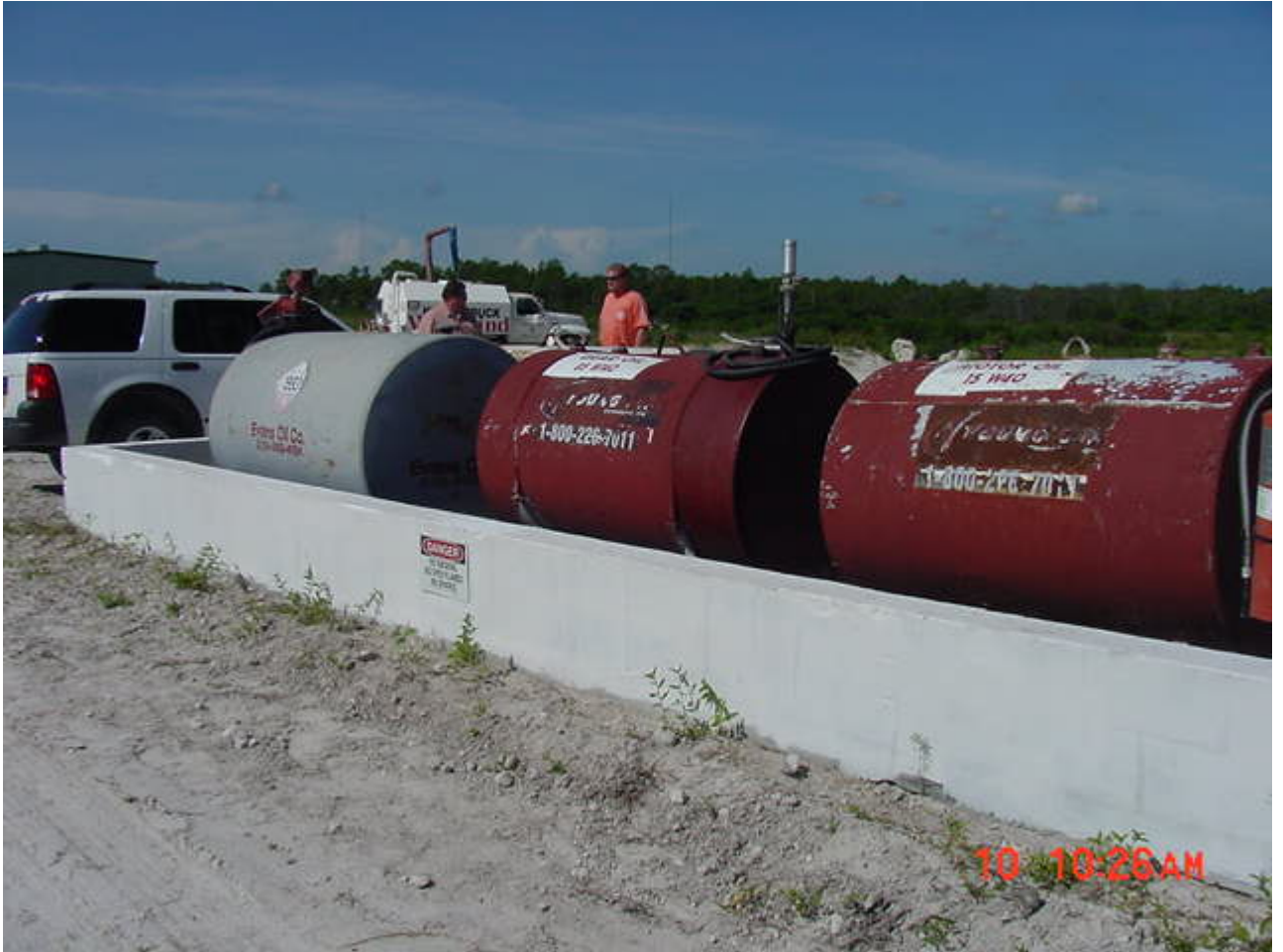
Other fuel tanks stored within containment system that holds the used oil tank. No roof over the containment system to protect from weather.
